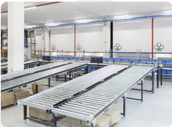
CONVEYOR BELTS AND ROLLER UNITS
