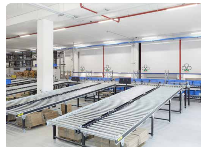
CONVEYOR BELTS AND ROLLER UNITS
